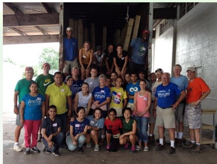
Members of the Habitat Young Professionals held a wall build in August to officially kick off the construction of the Young Professionals Habitat house.
